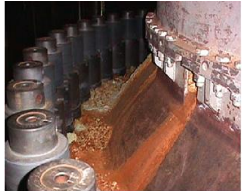
Accidental Boric Acid Corrosion at RPV outer surface
